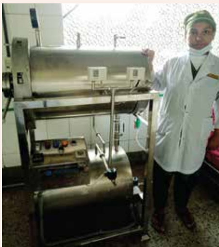
Fig. 22. Newly installed Autoclave in 214 ward, Obs. & Gynae. Department.
